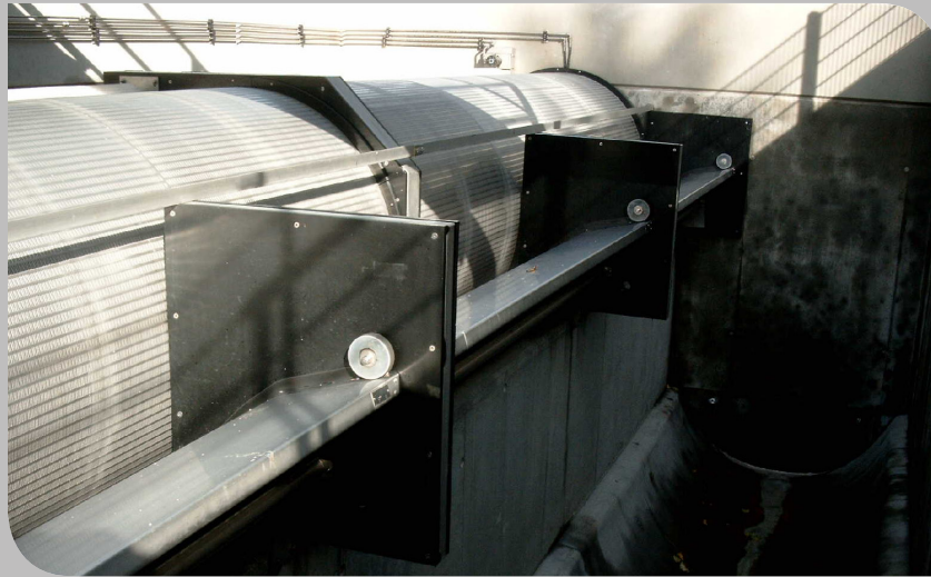
Figure 2: Hydraulic optimization using the HYDROVEX® BW Bending Weir with the HYDROVEX® RDS
